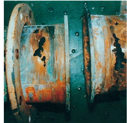
DAMAGES OF A COPPER NICKEL PIPE AFTER SIX MONTH BECAUSE OF NON INSULATION
